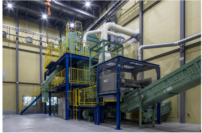
Vertical crusher installed at the third plant
