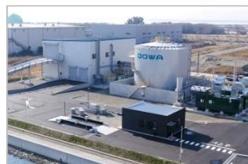
The biogas power generation plant
