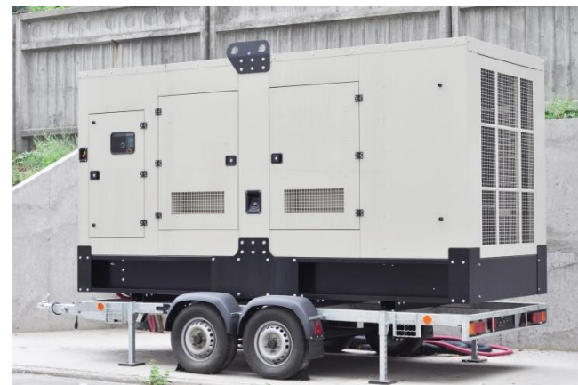
Emergency power supply
