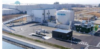
Biogas power generation plant
