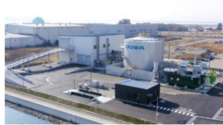
Biogas power generation plant
