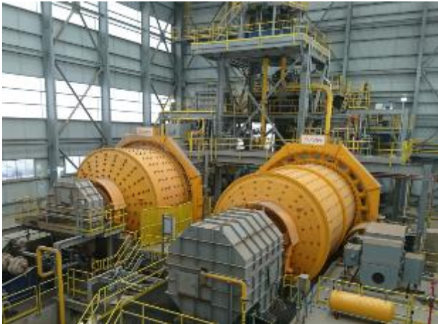
Ore crushing equipment at the Los Gatos Mine
