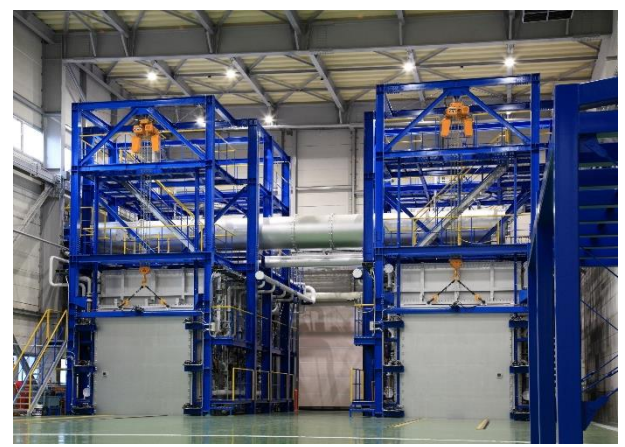
Heat treatment facility in Akita
