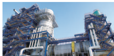
Waste incinerator, Eco-System Chiba Co., Ltd.
