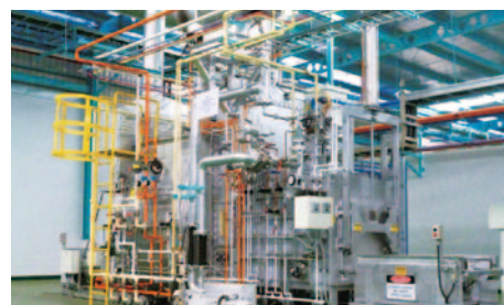
Industrial furnace installed at our base in Indonesia
