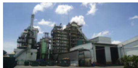
Waste treatment facility in Thailand
