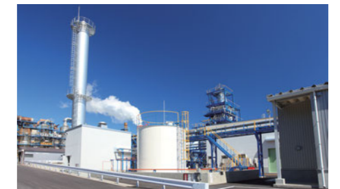
ECO-SYSTEM AKITA's low-contaminated PCB waste treatment facility
